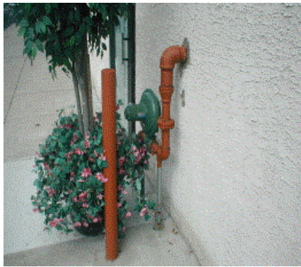
High Pressure Service Installed Outside Protected By Bollard & Hidden By Planter
